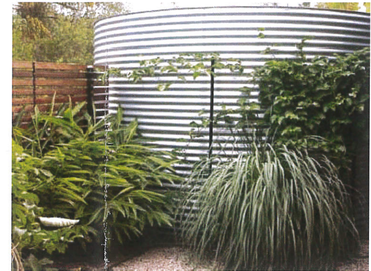
RAINWATER STORAGE TANK
