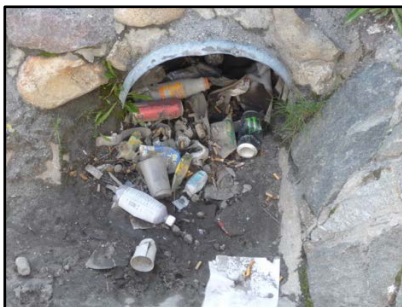
Image 1: Litter adds up and can clog culverts causing flooding
