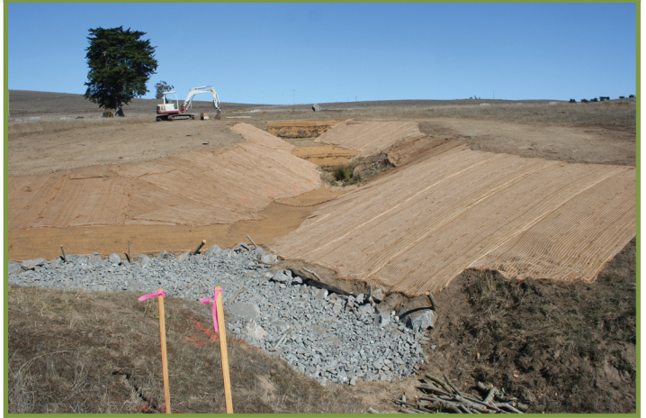
Marin Coast Ranch: DURING PROJECT, 2014 Grade Stabilization Rock Weir & Fabric Reinforced Earth Fill
